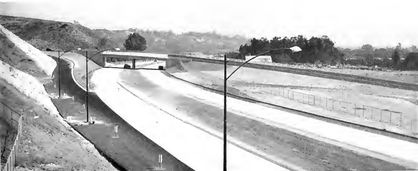
Looking easterly along Ramana Freeway showing Ganessa Avenue Overcrossing Bridge and westbound inlet ramp. Ganessa Park in background.
